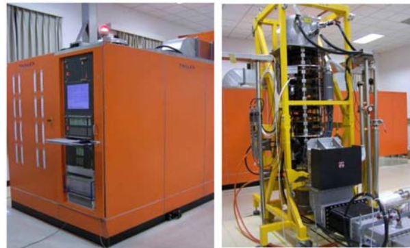
Fig. 6. The PSM power supply with an EPICS-based control panel (left); klystron (right).
